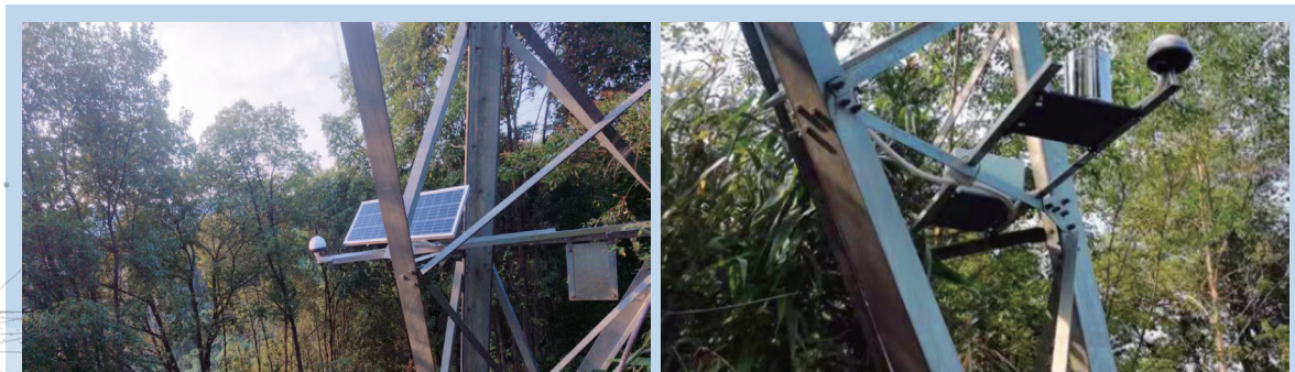
Hi-Target tower monitoring system equipment mounted on towers FIG5
